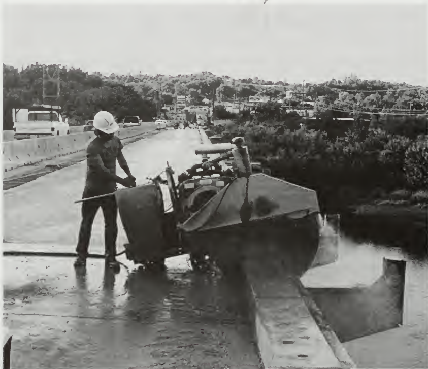
The giant saw blade used in this heavy construction work is edged with diamonds. Courtesy of CIMLINE Company.
