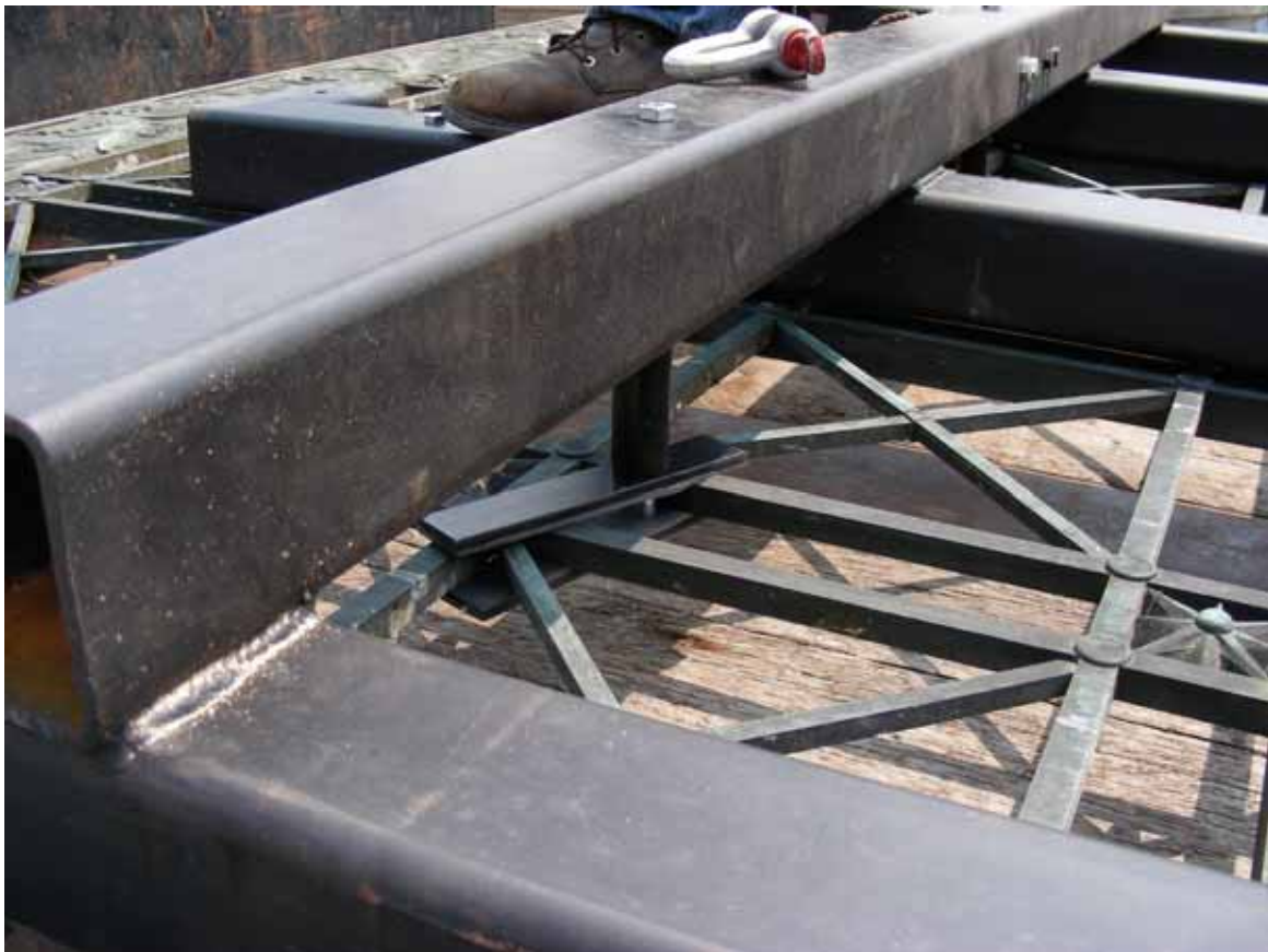
Figure C4. Steel bracing for removal of bronze grilles in 2007. Photograph courtesy of Melissa S. Meighan, PMA.
