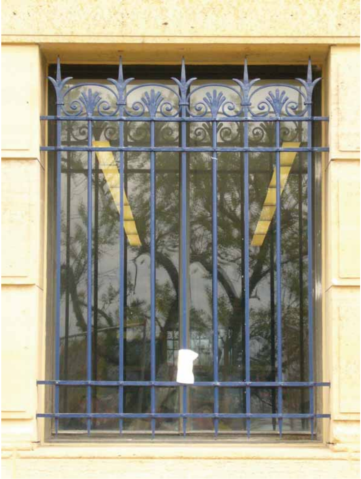
Figure C3. Treated and repainted iron grilles reinstalled at the PMA. Photograph taken by author (April 2008).
