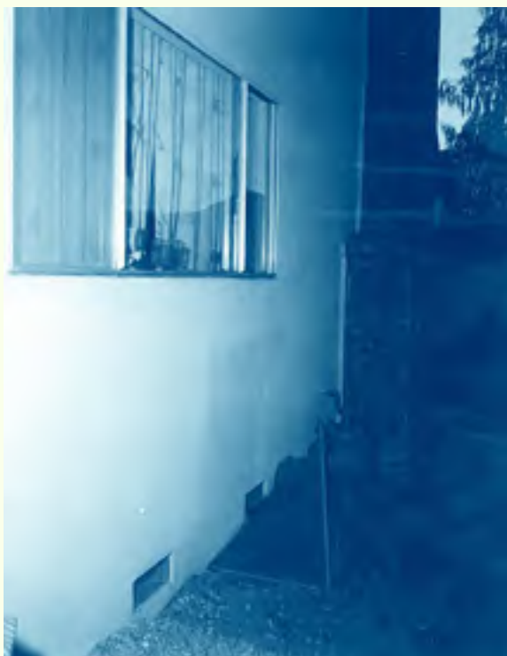
FIGURE 37—The windows in many older buildings were constructed at a height that makes them too easily accessible from the ground.
