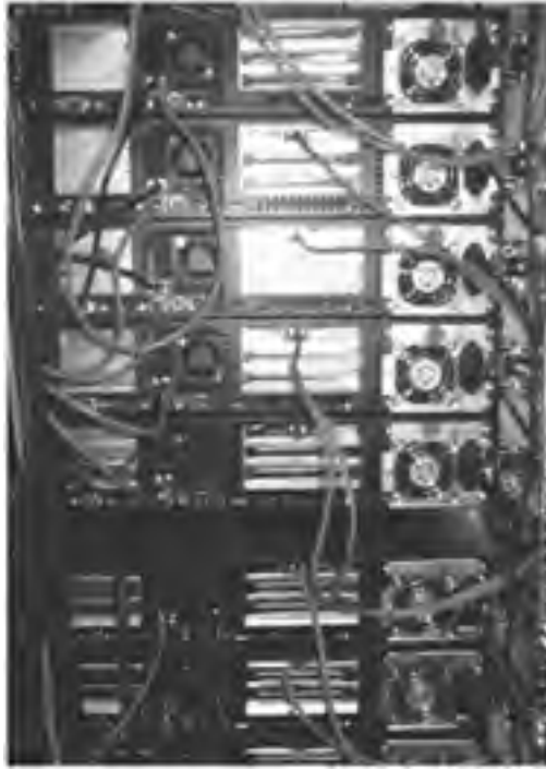
Figure 6.2: The back of a rack, showing the clean organization of the cables. Note that the fans are unobstructed.
